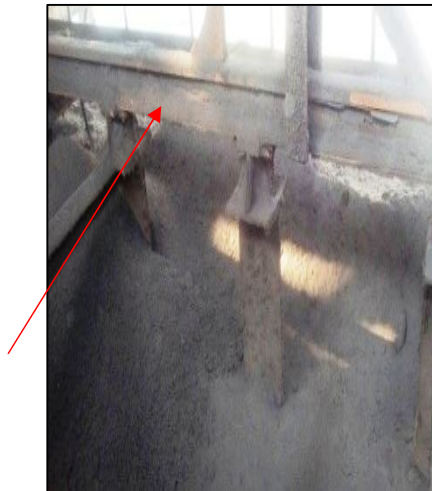
Heavy deposition of dust & corrosion noted on the member
