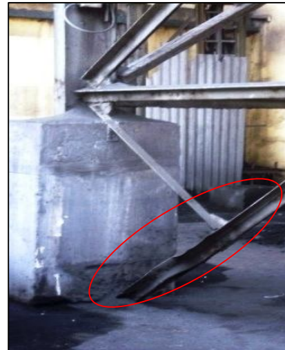
Noted bent cross bracing with corrosion
