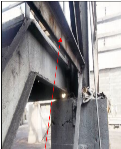
Corrosion in horizontal bracing
