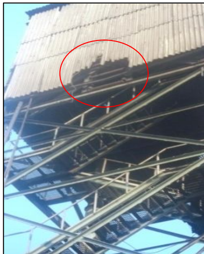
A.C sheet broken/ damaged
