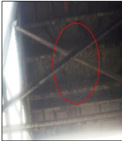
Sever corrosion & deposition of dust on the all the members
